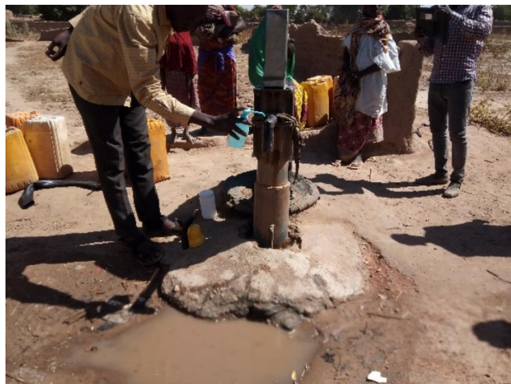
Photo 5: Poor well head construction Drainage around Hand Pump
